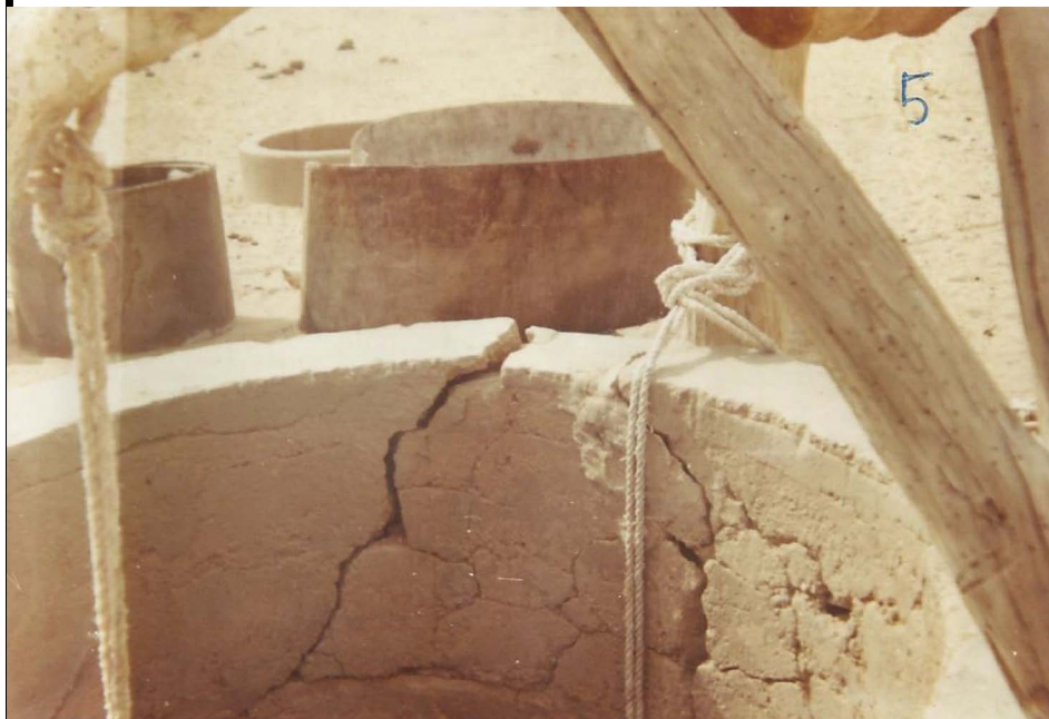
FON Provides Funds for Well Repair in Touloukh Top: Before Repair; Bottom: After Repair
