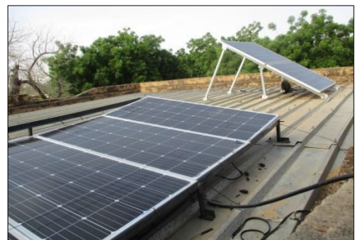
Solar panels – Yekoua Health Clinic
